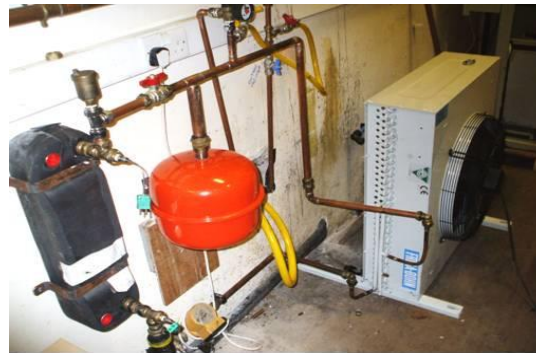
Figure 15. The connections of the heat exchanger, water pump, heat rejection fan and expansion valve
