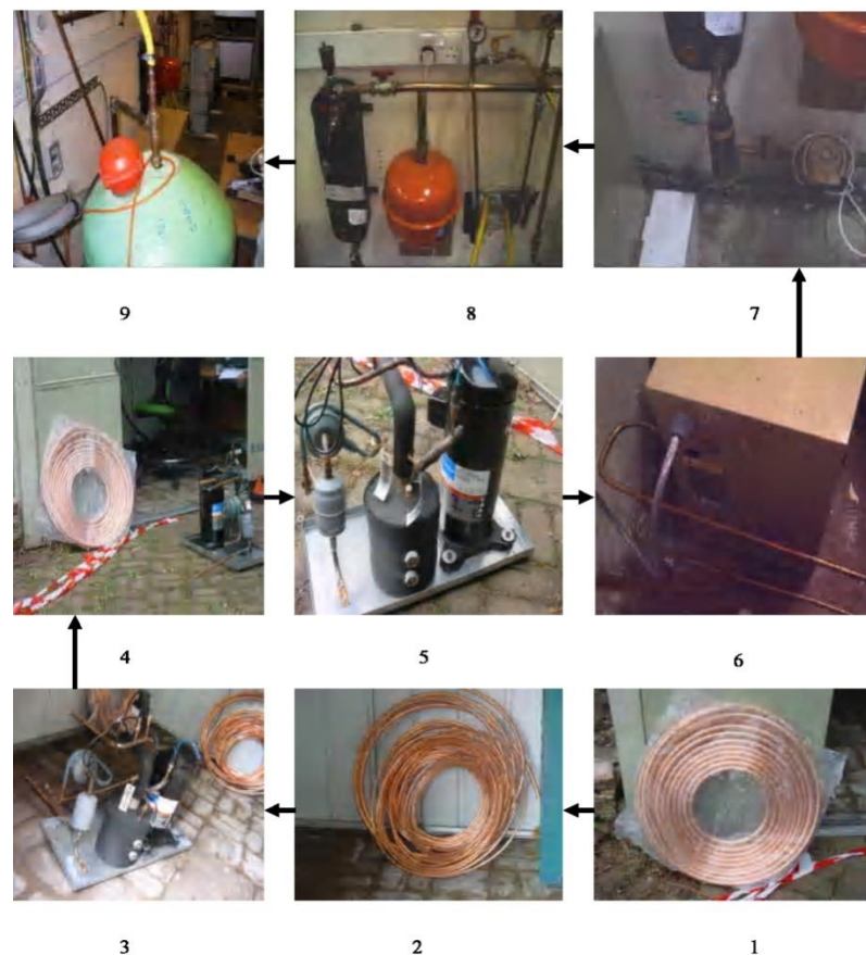
Figure 4. Preparation of coils (1-2), installation of heat pump (3-6) and connection of water supply system (water pump, flow meter, expansion valve and the boiler) (7-9)
