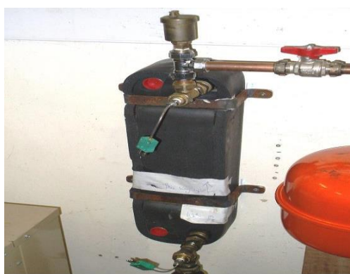
Figure 14. The heat exchanger
